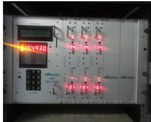
Data logger front end Processor at DRM's Office Bhavnagar
